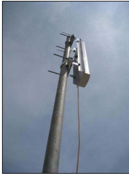
Figure 7 : WBA antenna mounted on pole.
